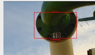
ANOMALY DETECTION, BOLTS ARE MISSING
